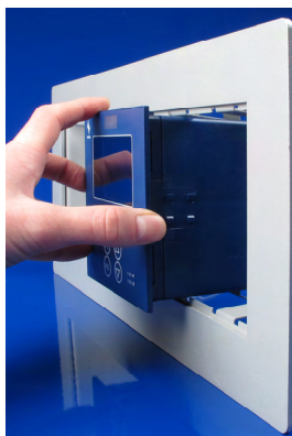
Installation in the MGR
