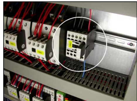
Wiring of a safety coil with RC combination
